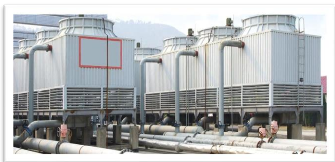
Representative picture of Industrial cooling water towers
