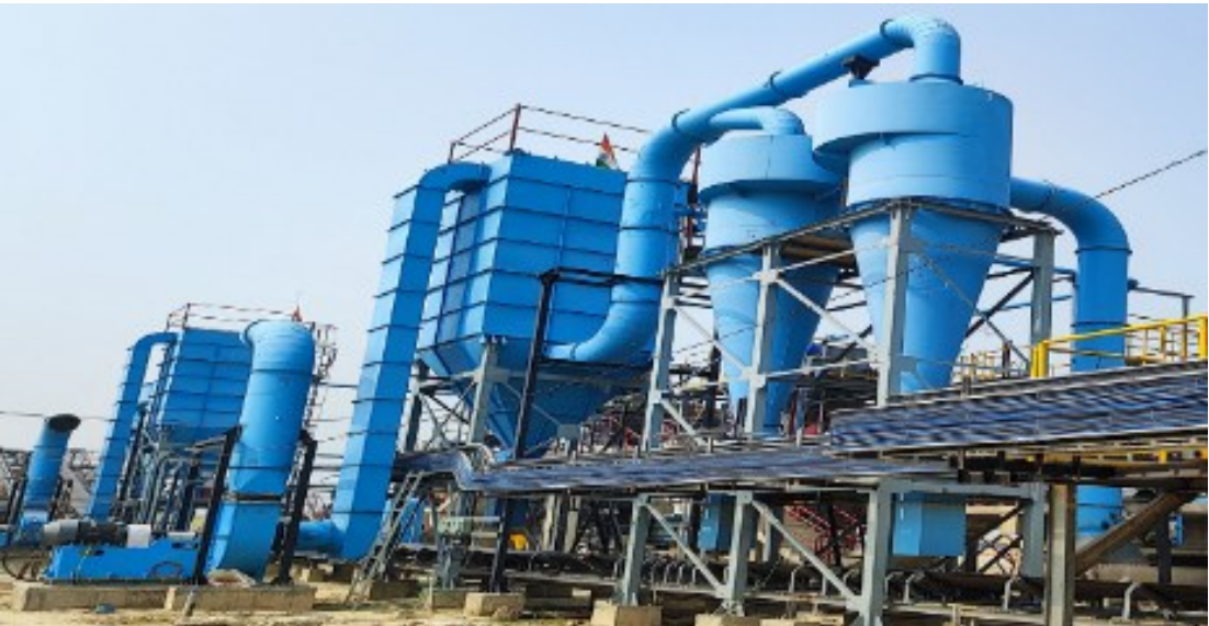
CBG Plant at Budaun- Milling Section
