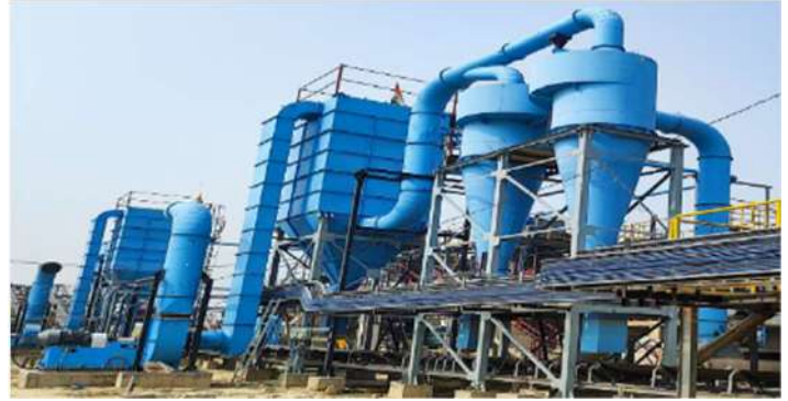
CBG Plant at Budaun- Milling Section
