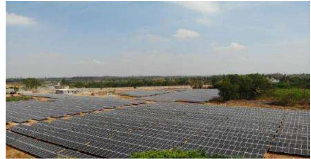
Solar Panels at HRGRDC, Bengaluru
